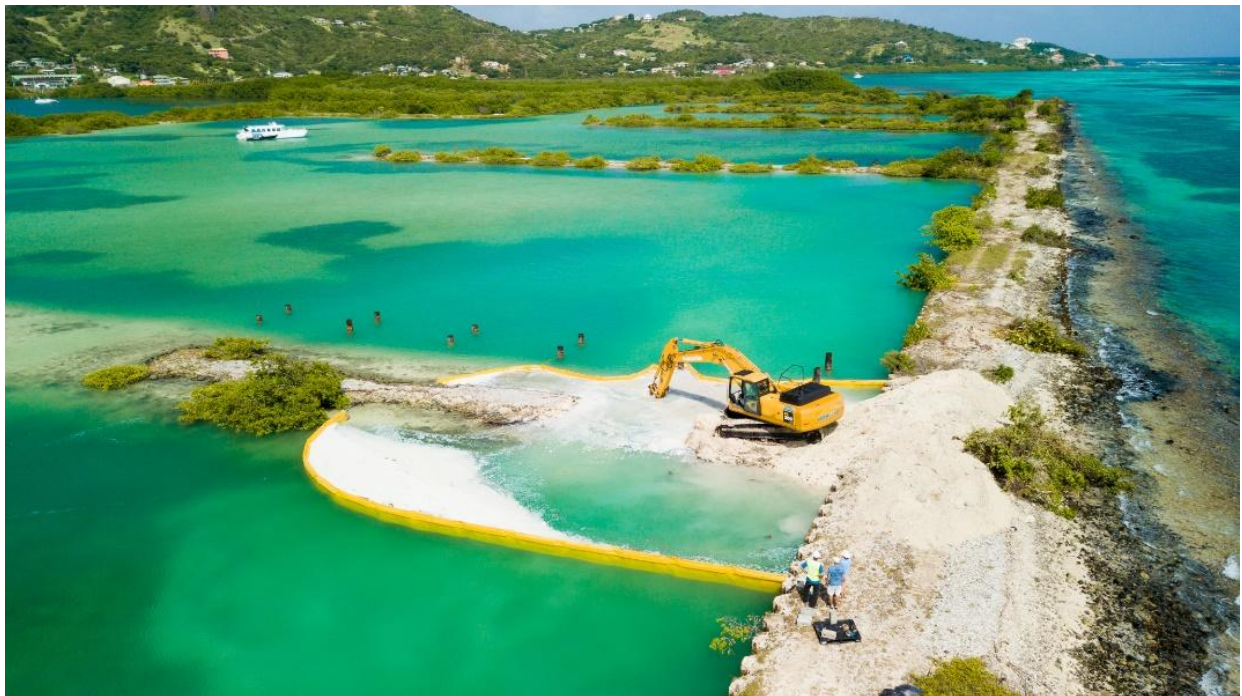
Excavation at gap 2. Turbidity barriers were deployed to prevent sediment from harming marine life. Photo credit: Arthur Daniel.
